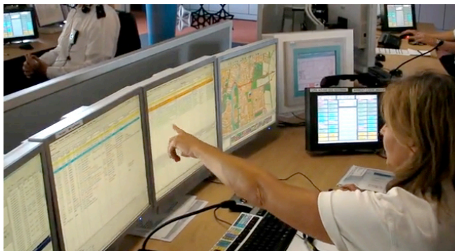
Figure 1 - Control Room at VRK, Haarlem, NL
